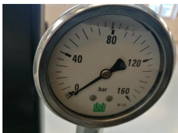
Abb. 10 The gauge for showing the pressure of the system
